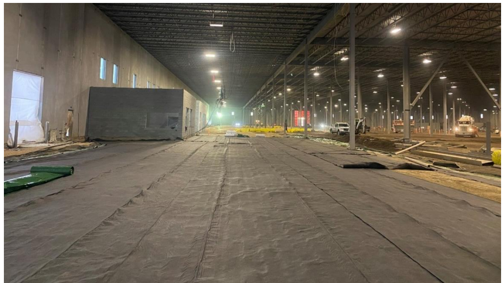
Commercial Warehouse Building in a Radon Gas sensitive area in Edmonton, Canada
