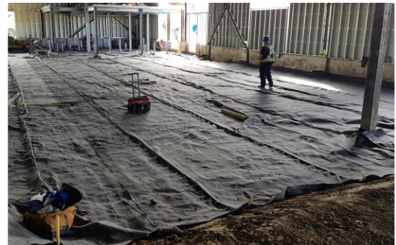
Installation of DRAINTUBE GAS as part of the Sub-slab Depressurization System (SSD).
