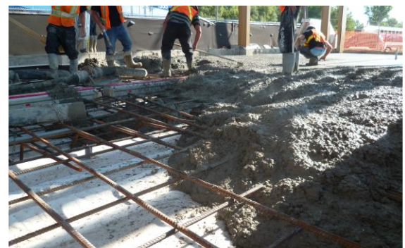
Pouring the concrete slab on the DRAINTUBE 500P FTB1 D25. The needle punched geofilm on top of the product prevents migration of the fresh concrete into the geocomposite.
