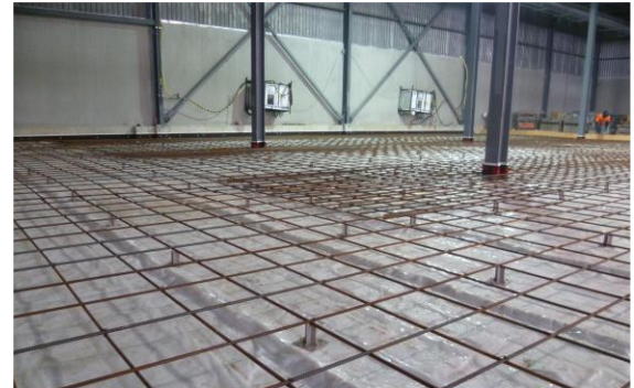
Installation of DRAINTUBE 500P FTB1 D25 as part of the subslab depressurization system.
