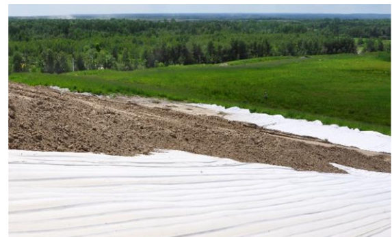
Backfill placement on the DRAINTUBE®. The geocomposite protects the geomembrane against puncture from the surrounding soil layers.
