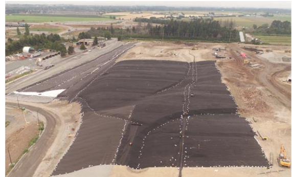
Installation of DRAINTUBE 606 ST2 D25 for gas venting below the liner. Each DRAINTUBE® panel is mechanically connected to a main header using the Quick Connect System.
