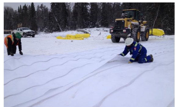
Installation of DRAINTUBE 400P FT1 D25 in winter. Low bearing capacity residues show better resistance when frozen at -25°C (-15°F).
