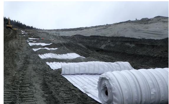
DRAINTUBE 300P FT4 D25 is used in strips into the cycloned sand dam for pore pressure release and stability increase.
