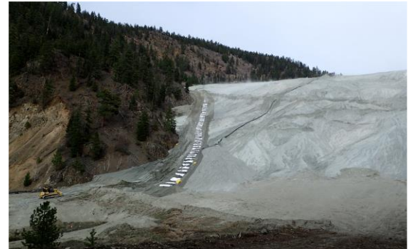
Installation of DRAINTUBE 300P FT4 D25 as finger drain into the cycloned sand of a tailings dam.
