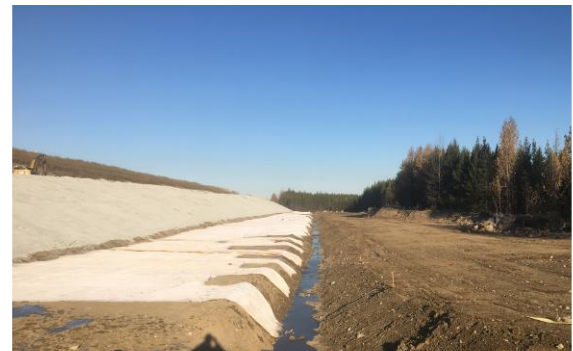
DRAINTUBE 300P FT4 D25 is installed at the base of the Dam to intercept water and control internal erosion.
