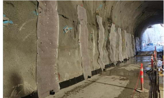
Strips of ALVEODRAIN EV mechanically fixed on the tunnel walls for vertical drainage.
