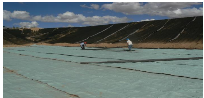
Figure 4: Installation of drainage geocomposites on the bottom of the test pool and placement of the collectors.
